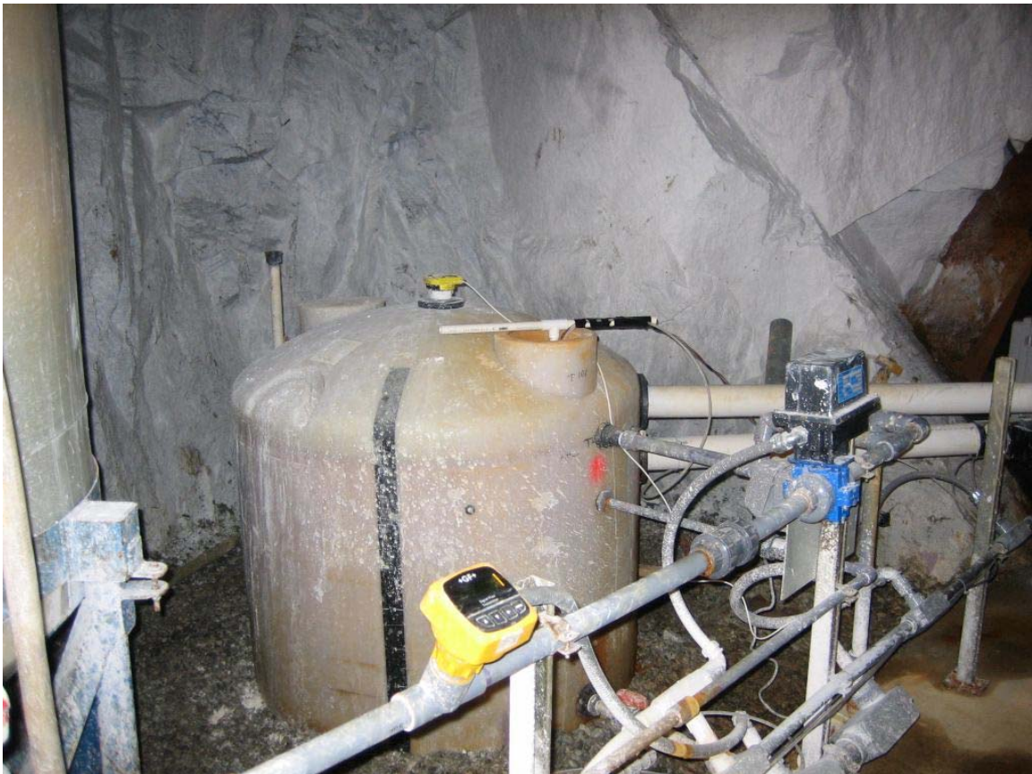
Figure 25. Inlet - Sample point 1.
