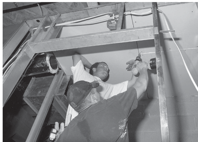
Because drywall is heavy and cumbersome, a helper generally assists the installer in positioning and securing the panel.
