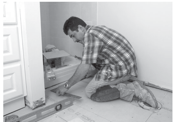
Prior to installing tile, tilers use measuring devices and levels to ensure that the tile is placed in a consistent manner.
