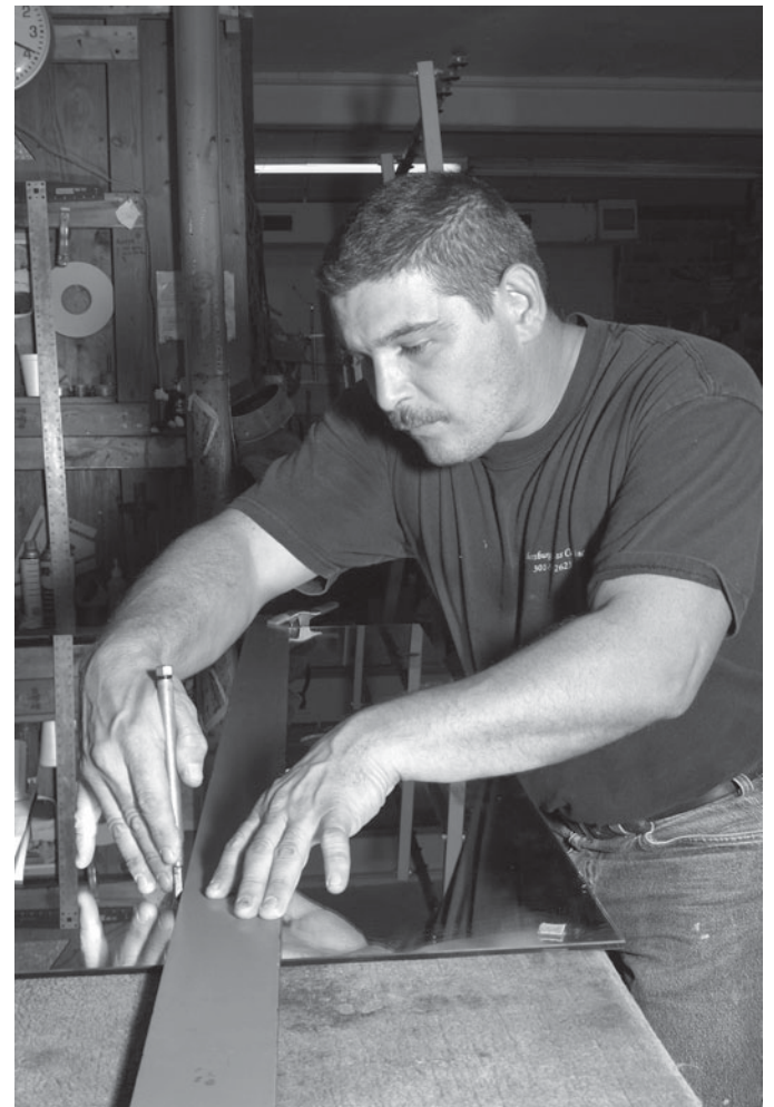
For some jobs, the glazier must cut the glass manually at the jobsite.
