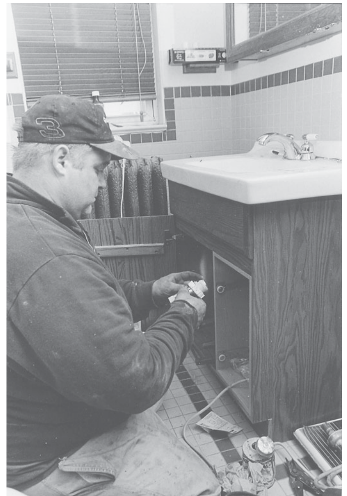
Pipelayers, plumbers, pipefitters, and steamfitters use many different materials and construction techniques, depending on the type of project.
