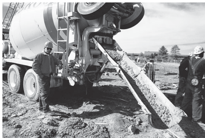
Sometimes, cement masons perform all the steps of laying concrete, including the finishing.
