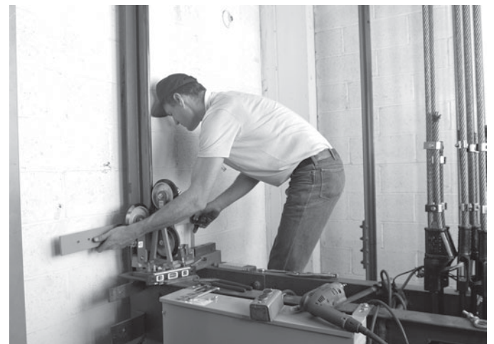
Once an elevator is operating properly, it must be maintained and serviced regularly to keep it in safe working condition.
