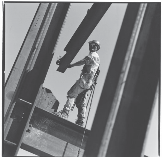
Even though the primary metal involved in this work is steel, these workers often are known as ironworkers .
