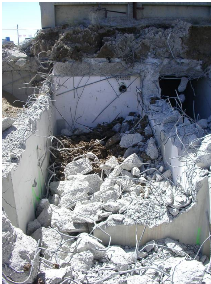
Figure B-2. Basement areas near B219, CV and ECCS building Ready for backfill.
