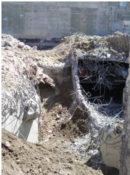
Figure 6. Process TAN-650 single level structures and -650 basement areas around CV to three feet before grade and dispose.
