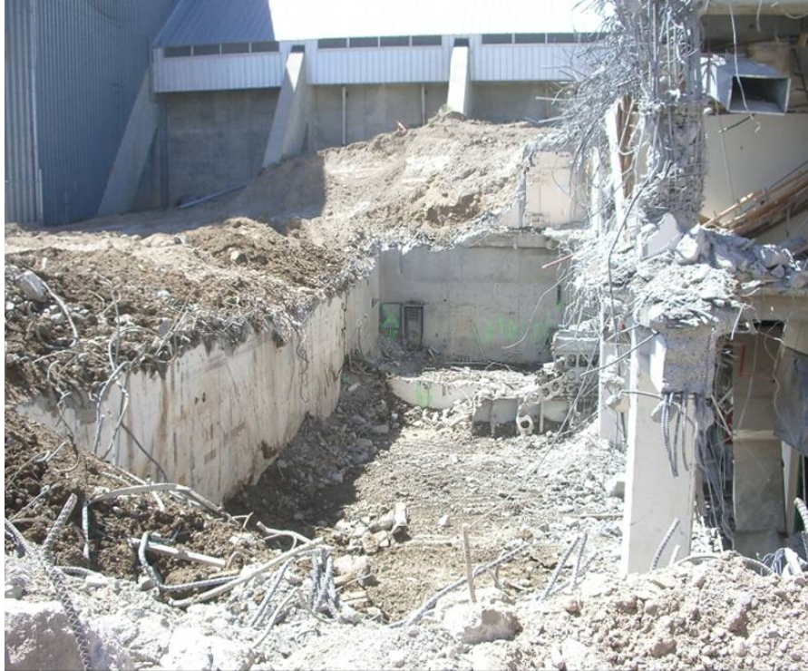
Figure B-17. South and Southeast portion of B101 area ready for partial backfill.
