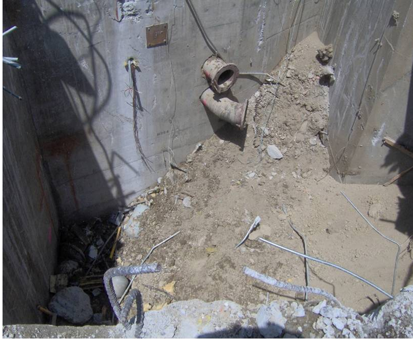
Figure B-21. East portion of CV area Rm B224/225 ready for backfill.
