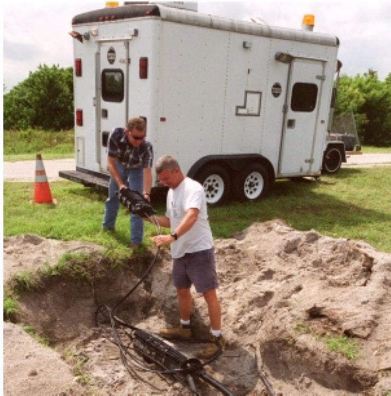
At left, United Space Alliance (USA) communication engineers, Larry Wages, left, and Phil Adams, bury fiber optic connectors for KSC's complex communication system. Below, USA overhead crane operators Lonnie Watson, left, and Richard Welch work in the bridge cab on the 34th level of the Vehicle Assembly Building.
