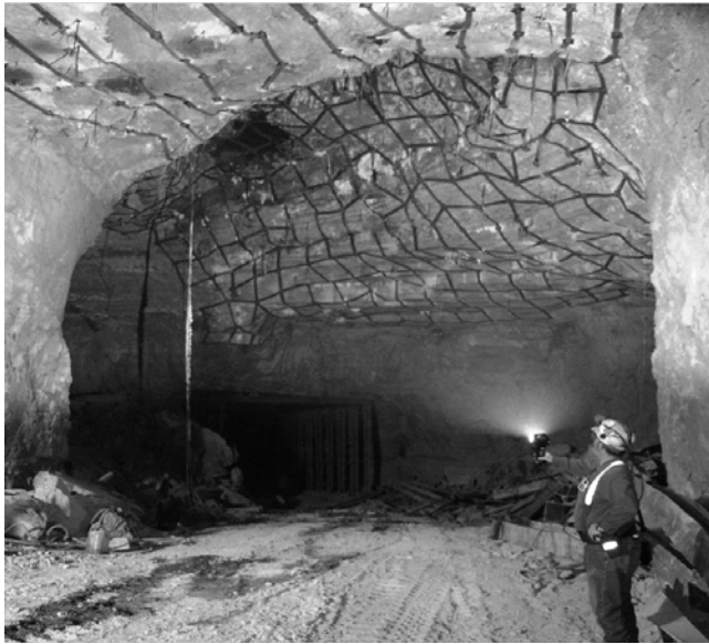
Figure 4. Repair of a large roof fall in which horizontal stress is thought to have contributed to the failure.
