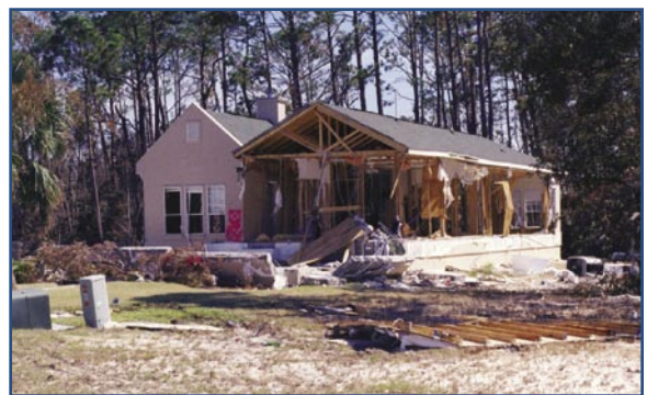
Figure 4. Compliant building damaged when the flood elevation exceeded the BFE.
