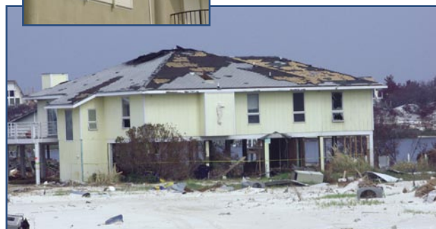
Figure 2. Well-sited buildings that still sustained damage due to building envelope and connection failures.
