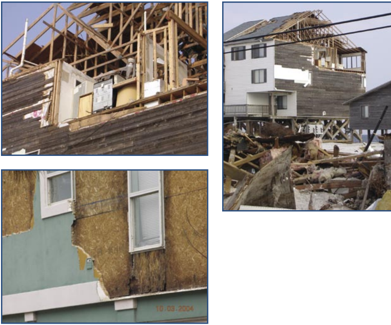
Figure 3. Well-sited building that still sustained damage due to building envelope and connection failures.
