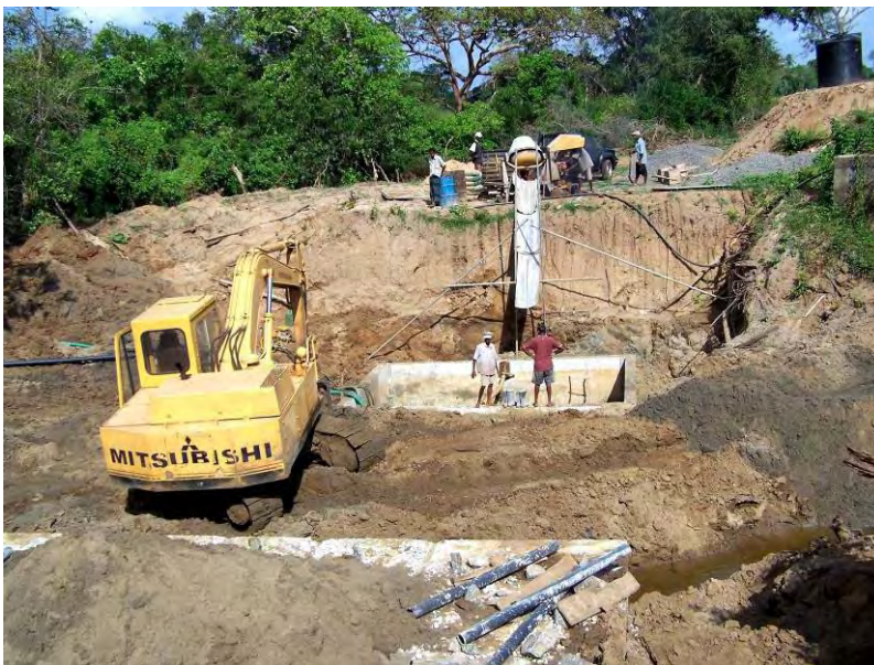
DAIC615 - Construction of a bridge reconnecting communities, improving economic opportunities and access to facilities begins
