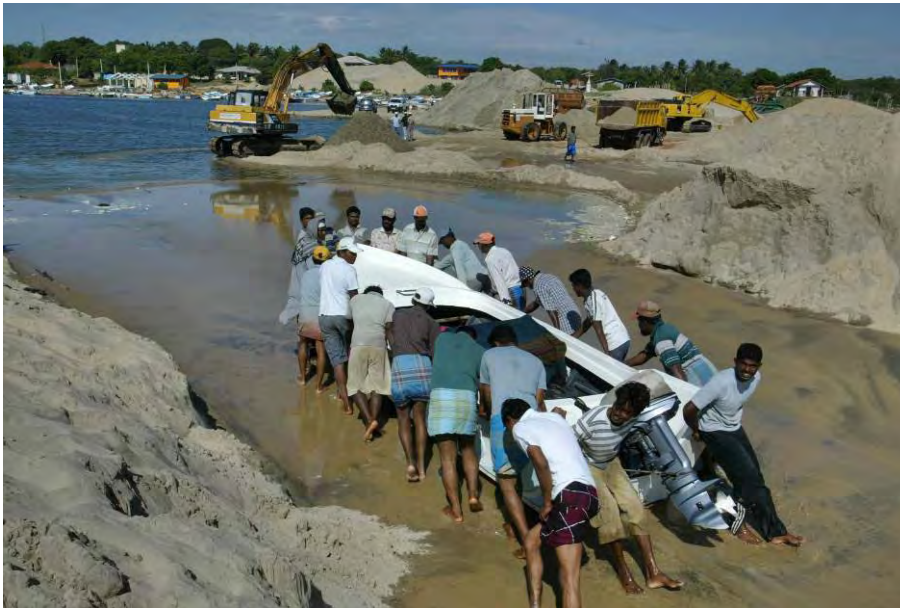
The tsunami dumped tons of sand in the Kirinda harbor and damaged the harbor’s dredger and excavator. Grant DAIC549 repaired these machines and supported the dredging of over 133,000 cubic meters of sand enabling 6,000 fishermen to use their harbor again. The harbor cooperation sells the sand (US$15 per cubic meter) to the road development authority to build roads.
