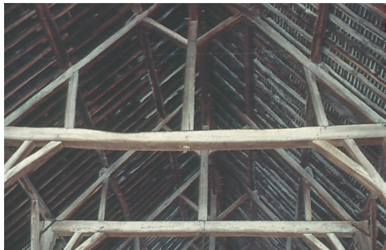
Fig. 3. Market hall, Milly-la-Forêt, 1479, with three-aisle basilican layout and double-framed "Latin Truss" roof with multiple purlins.
