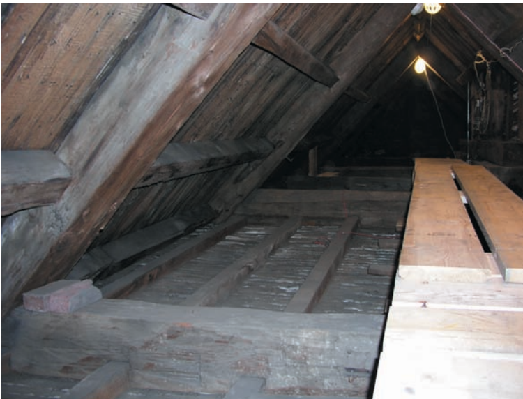
View under one side of the M-roof, with heavy collar beams carrying ceiling joists for the chambers below. Catwalk gives access to area seen in photo below.
