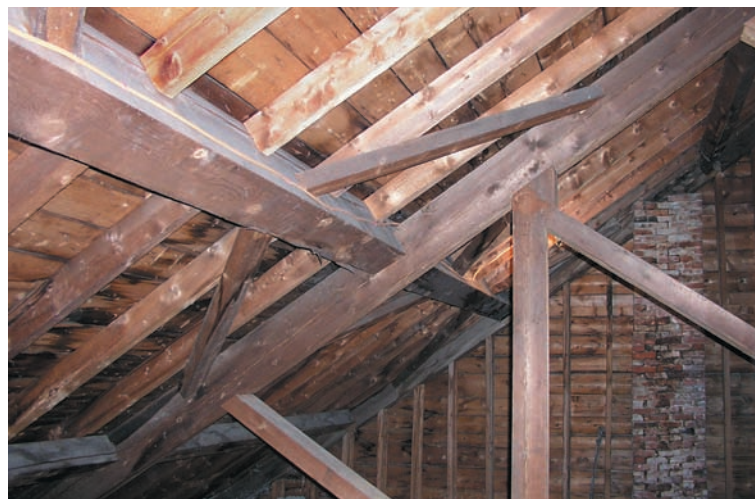
Huntington, upper part of truss with struted princepost. Wind-braced principal purlins overlap the upper chords and connect the trusses.
