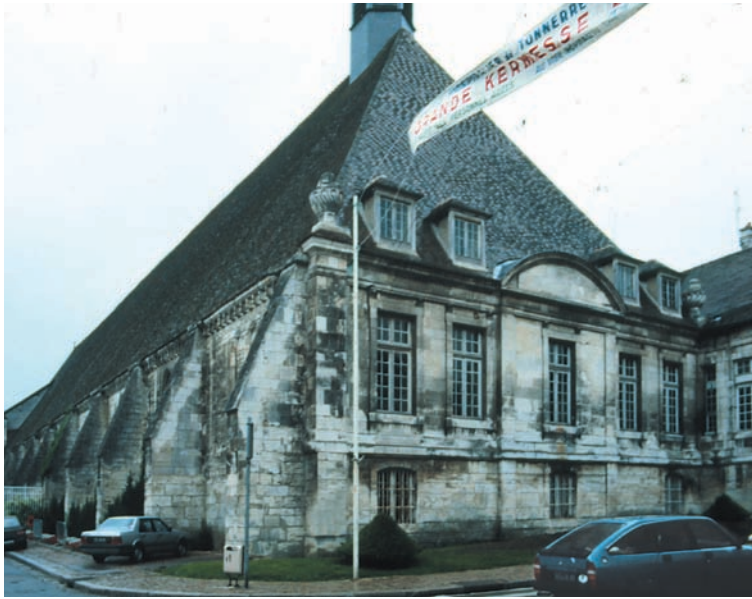
Fig. 13. The Maison Dieu in Tonnerre (1295). The vast roof, originally covered with glazed tiles, measures some 4500 sq. meters.
