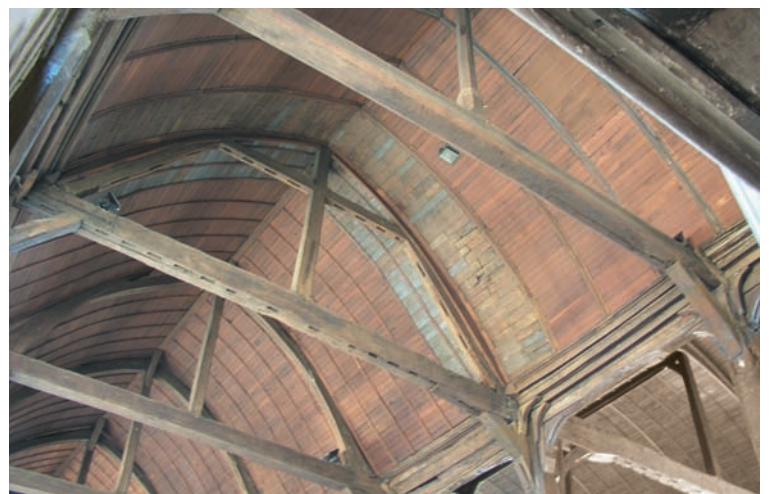
Fig. 12. One of two vaults at Ste. Catherine's. Empty mortises, patched lambrissée and change in rib centers indicate historic alteration.
