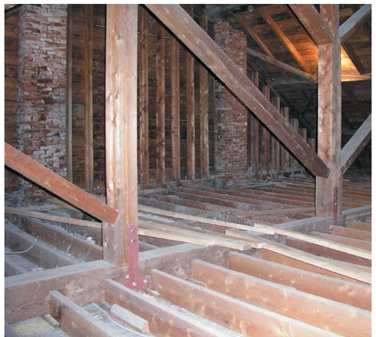
Lower part of truss. Toe-nailed 2x8 joists pass under the tie beams to set lath 2 in. below ties. Long-serving tension joints have been reinforced.
