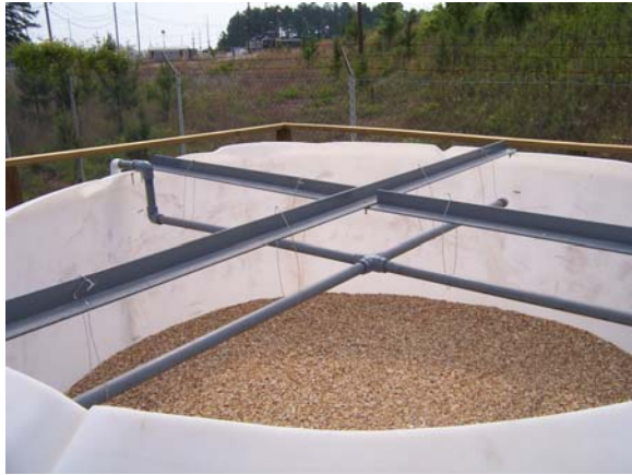
Figure 4. Influent distribution system on Tank 1
