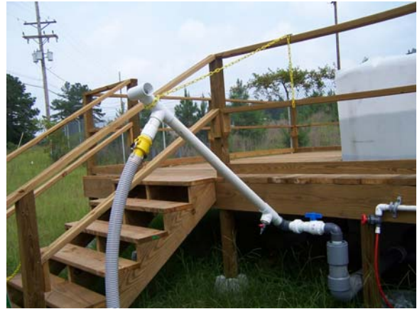
Figure 5. Effluent control arm with discharge tubing
