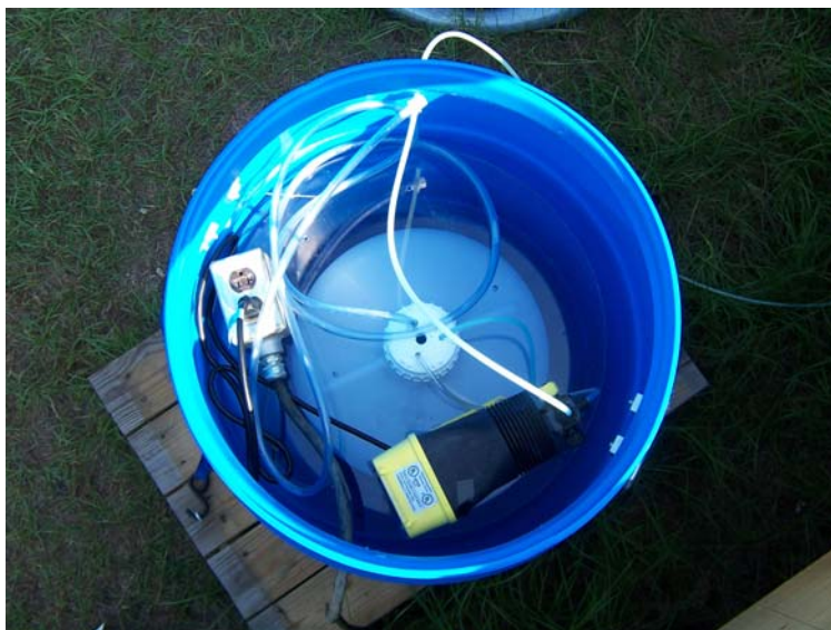
Figure 11. Chemical addition system
