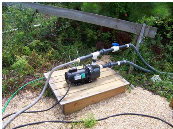
Figure 9. New water supply pump with overflow back to Outfall H-12
