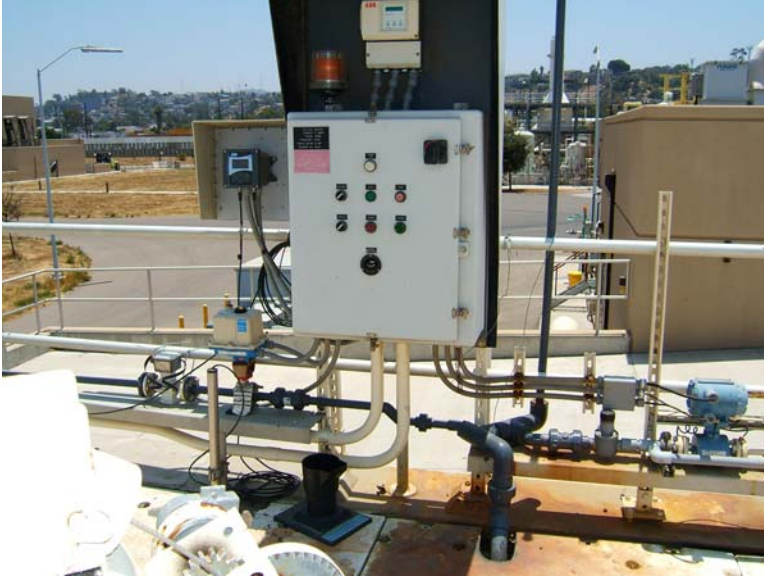
Ferric Chloride Dilution System for Grit Chamber
