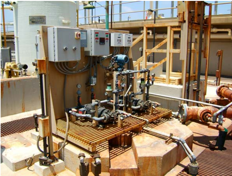
Ferric Chloride Feed Pumps for JB1
