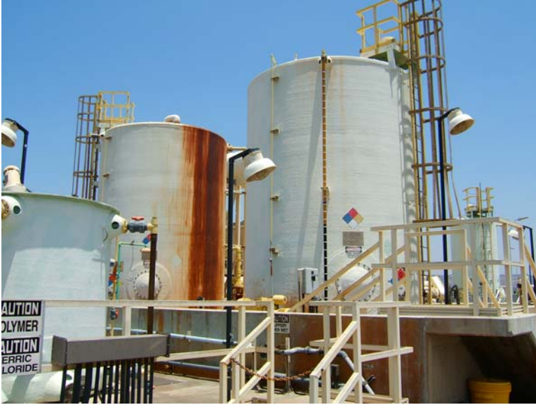
Ferric Chloride Tanks
