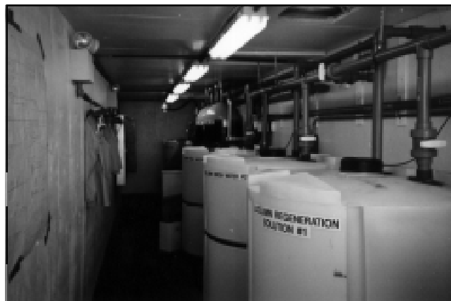
Ammonia Removal Processing Line
