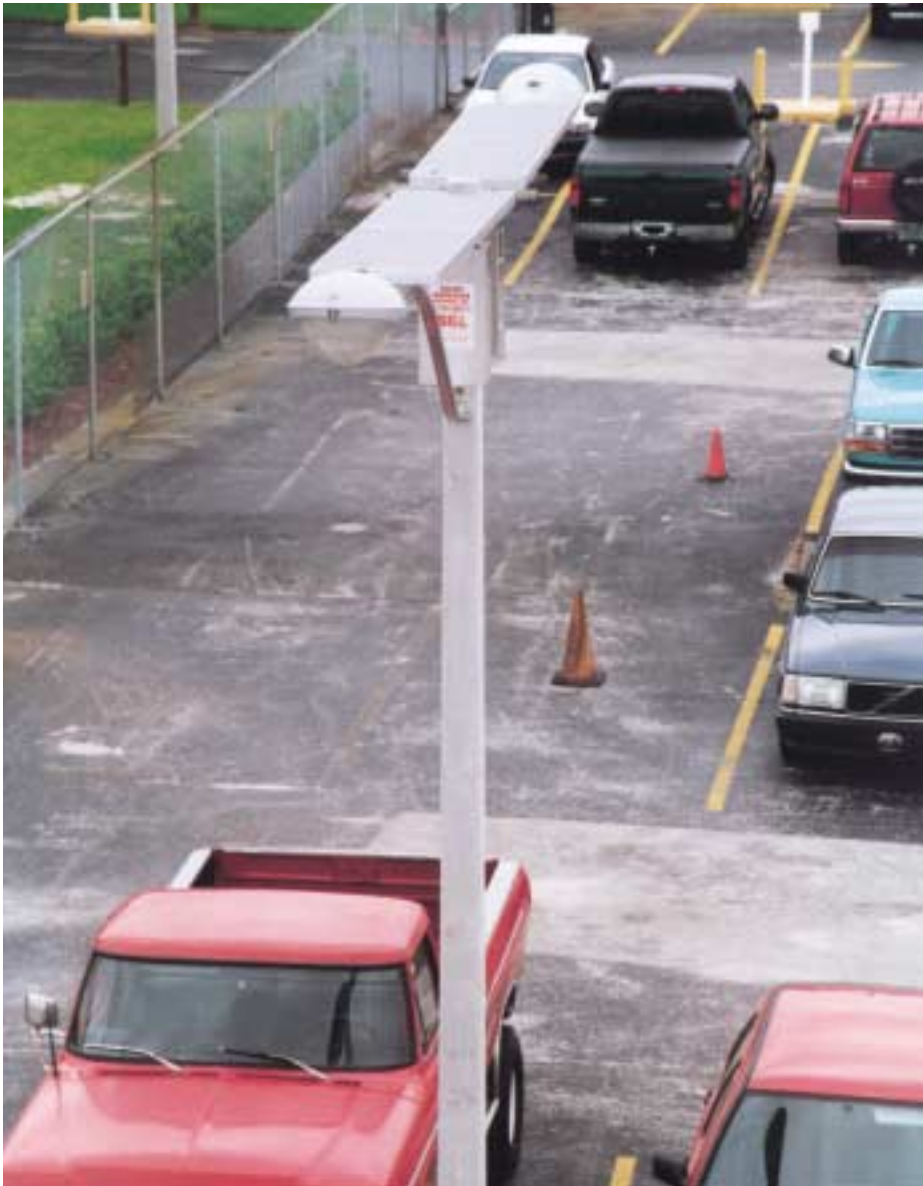
The flat, gray solar panels powering the parkinglot lights are hardly noticeable.
