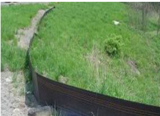
Photo 5, Silt Fence at a landfill. (SWANA, MOLO 2004, Ref. 4)
