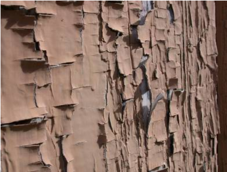
Photo 22. Lead based paint in deteriorated condition, Townsend 2004 (Ref. 28)
