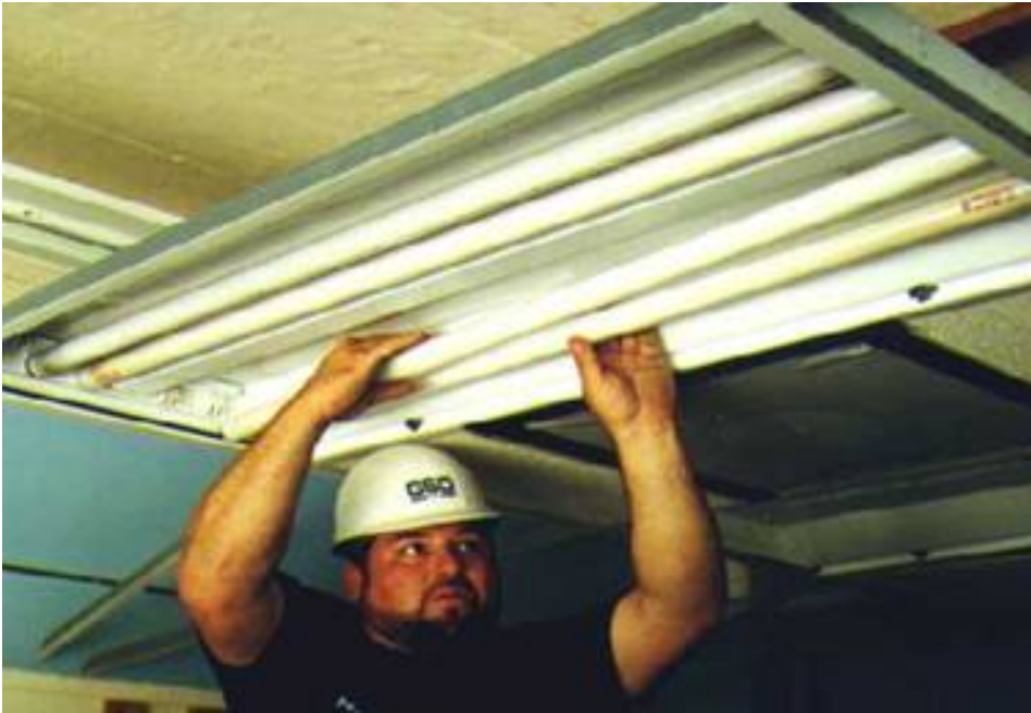
Photo 16. Typical Fluorescent Lamp Fixture , Townsend 2004 (Ref. 28)
