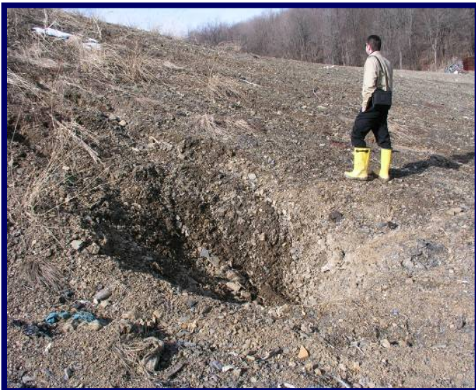
Photo 11. Depression caused by subsurface fire, 2004, Exit C&D landfill 1 (Landfill Fire Conference, Ohio EPA 2006, Ref. 17)
