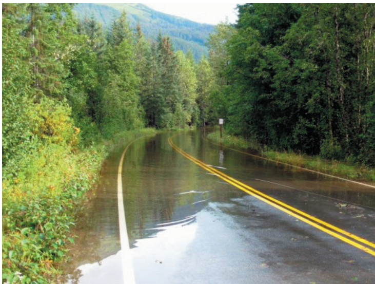
Flooding on Montana Creek Road in Juneau
