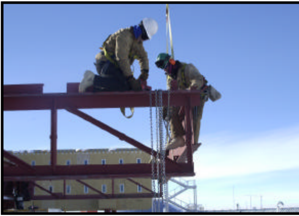
Left: Construction workers fix steel beams into place at the new Amundsen-Scott South Pole Station.
