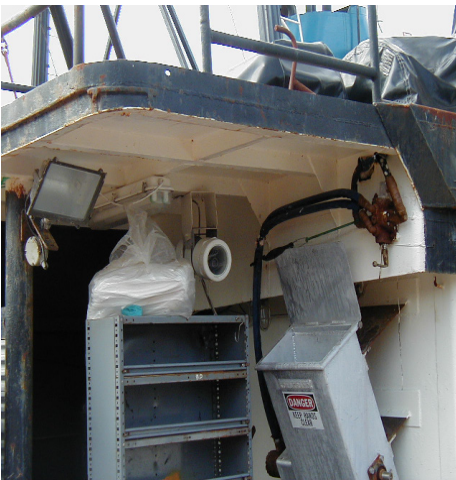
Figure 1: Closed-circuit TV camera (in the round white housing) and extra lighting at bait chopper
