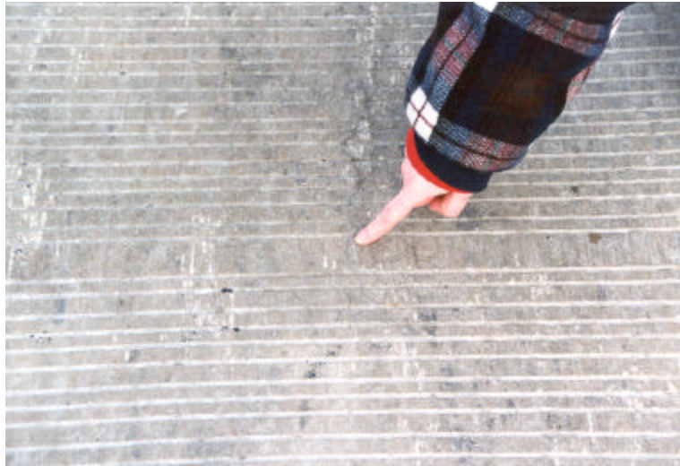
Photo 15. Longitudinal Crack (District 8 – Stage 1, Dec. 1, 1999)
