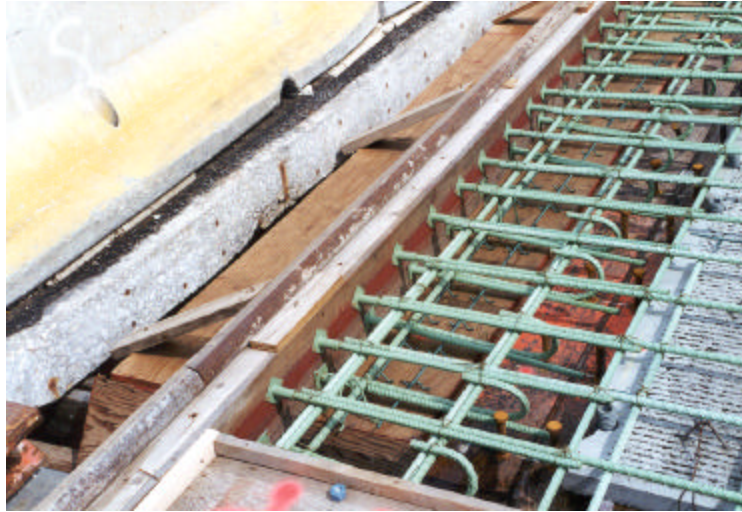
Photo 10. Bottom splice bars cut short (District 8 – Stage 1, June 24, 1999)
