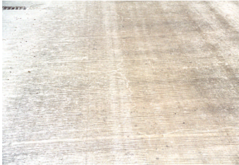
Photo 16. Longitudinal Crack (District 8 – Stage 1, January 28, 2000)
