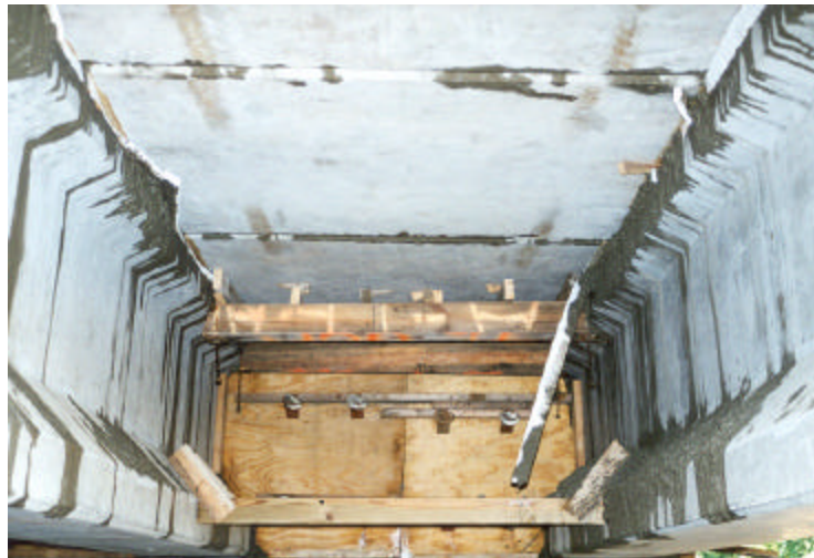
Photo 13. Blowouts (District 6 – Stage 1, August 16, 1999)
