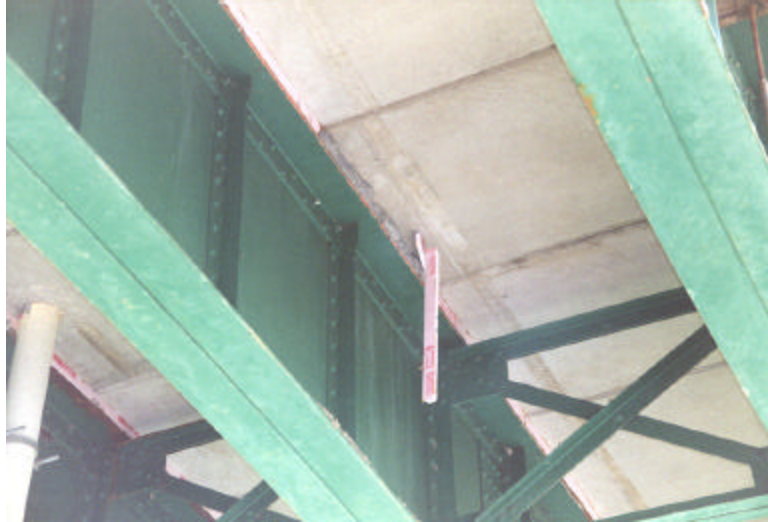
Photo 12. Blowout (District 8 - Stage I, June 28, 1999)
