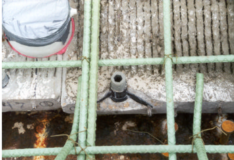
Photo 8. Spall at leveling insert (District 8 – Stage 1, June 24, 1999)
