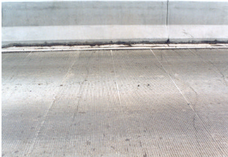
Photo 18. Transverse cracks above Pier #2 (District 6 – Stage 1 “creek” bridge, March 13, 2000)
