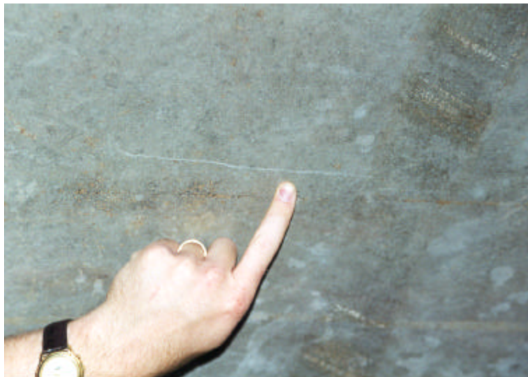
Photo 19. Crack on underside of PPC deck plank (District 6 – “overflow” bridge, May 30, 2000)
