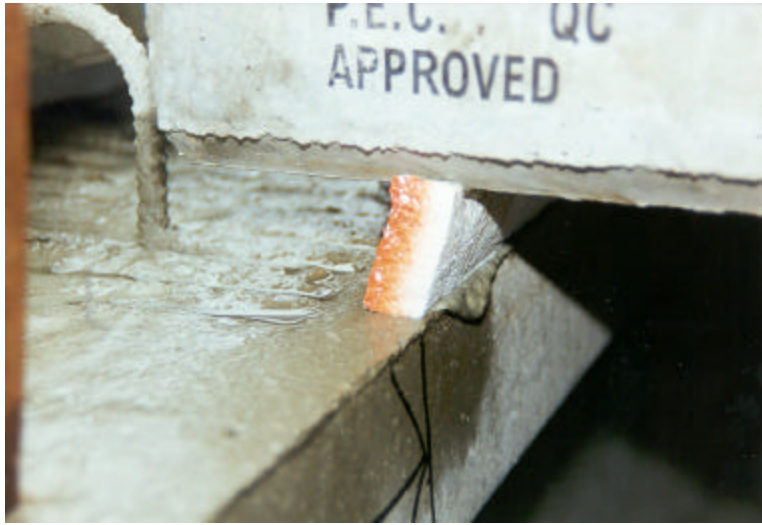
Photo 1. PPC deck plank seated on polystyrene (July 1999 – District 6)
