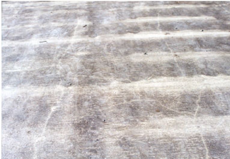
Photo 17. Longitudinal, transverse, & diagonal cracks before traffic loading (District 6 – Stage 1 “overflow” bridge, August 30, 1999)
