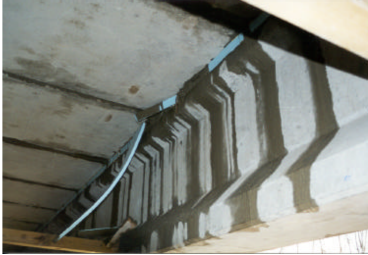
Photo 14. Blowouts (District 6 – Stage 2, March 13, 2000)
