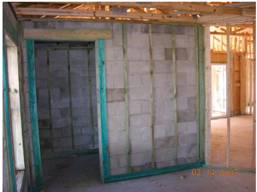
View of an in-residence shelter under construction. Steel reinforced and fully grouted CMU surround the shelter space.
