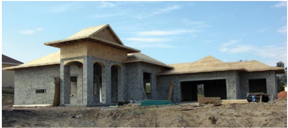
CMU was used for the exterior walls at this house under construction.
