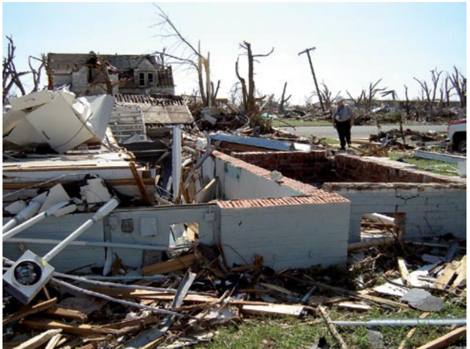
First floor of residence that shifted during a tornado, exposing the basement (Greensburg, KS).
