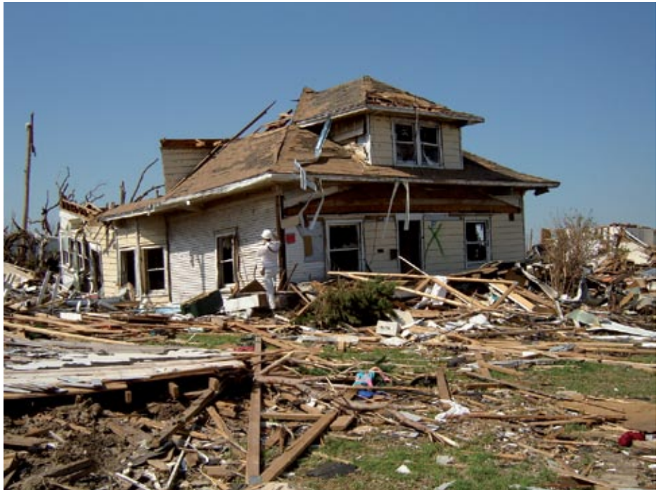
Residence that slid on its foundation and collapsed partially into the basement (Greensburg, KS).
