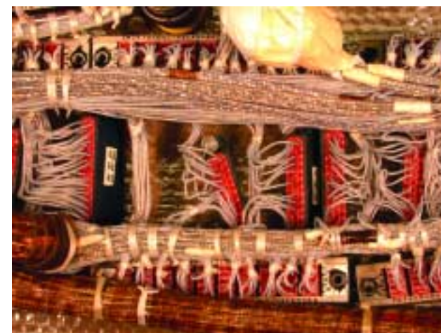
Close-up view of IEA shows intricacies of wiring.
