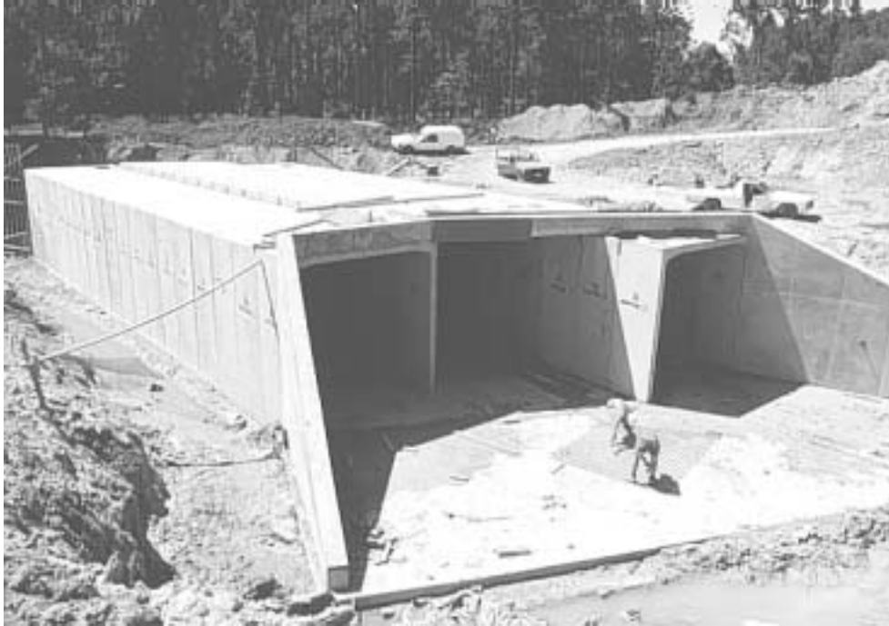
Figure 15. Concrete aprons are used to disperse water flow at the culvert outlet (Photo courtesy Main Roads Photo Visual Library).
