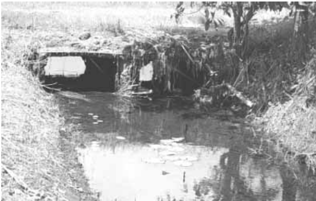
Figure 14. Crossing structures should be as wide as the stream to ensure that water flow is not restricted and water velocity is not increased. Tully, Queensland.
