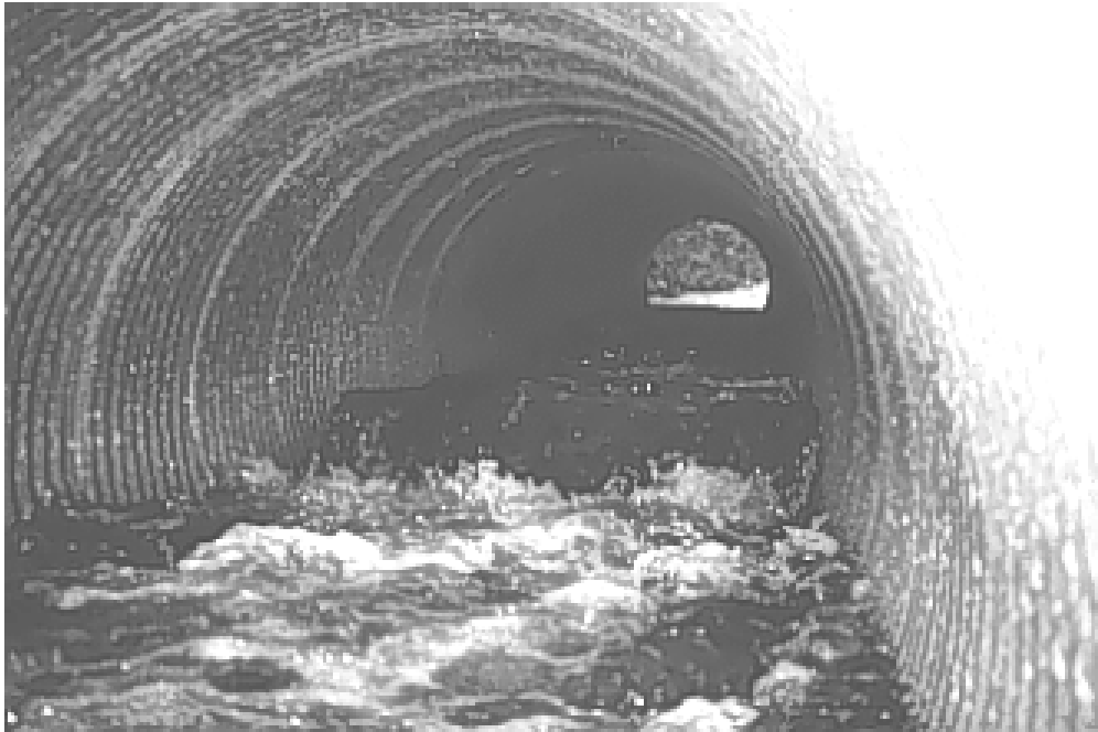
Figure 11. Baffles may be installed in culverts to increase barrel roughness and reduce water velocity (Photo courtesy K. Bates).
