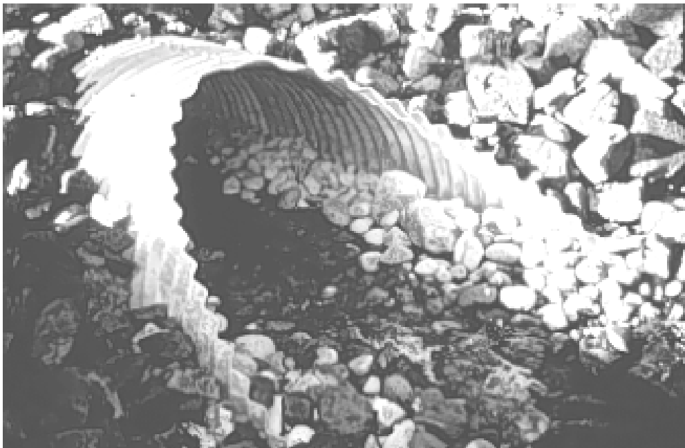
Figure 10. Placing rocks in the bottom of culverts can simulate the natural stream bed (Photo courtesy K. Bates).
