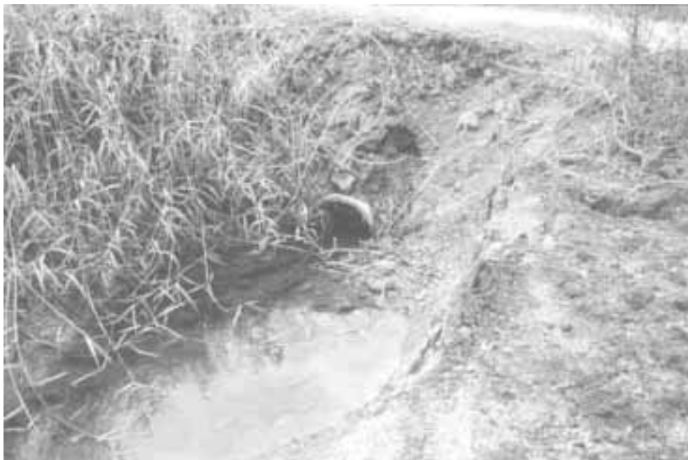
Figure 16. Culverts can become overgrown and clogged with sediment and/or debris if not regularly maintained. Tully, Queensland.
