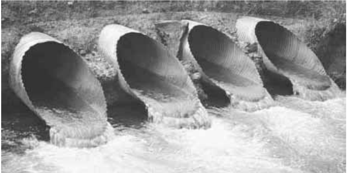
Figure 2. Series of pipe culverts where erosion has created a drop at the outlet. Tully, Queensland.
