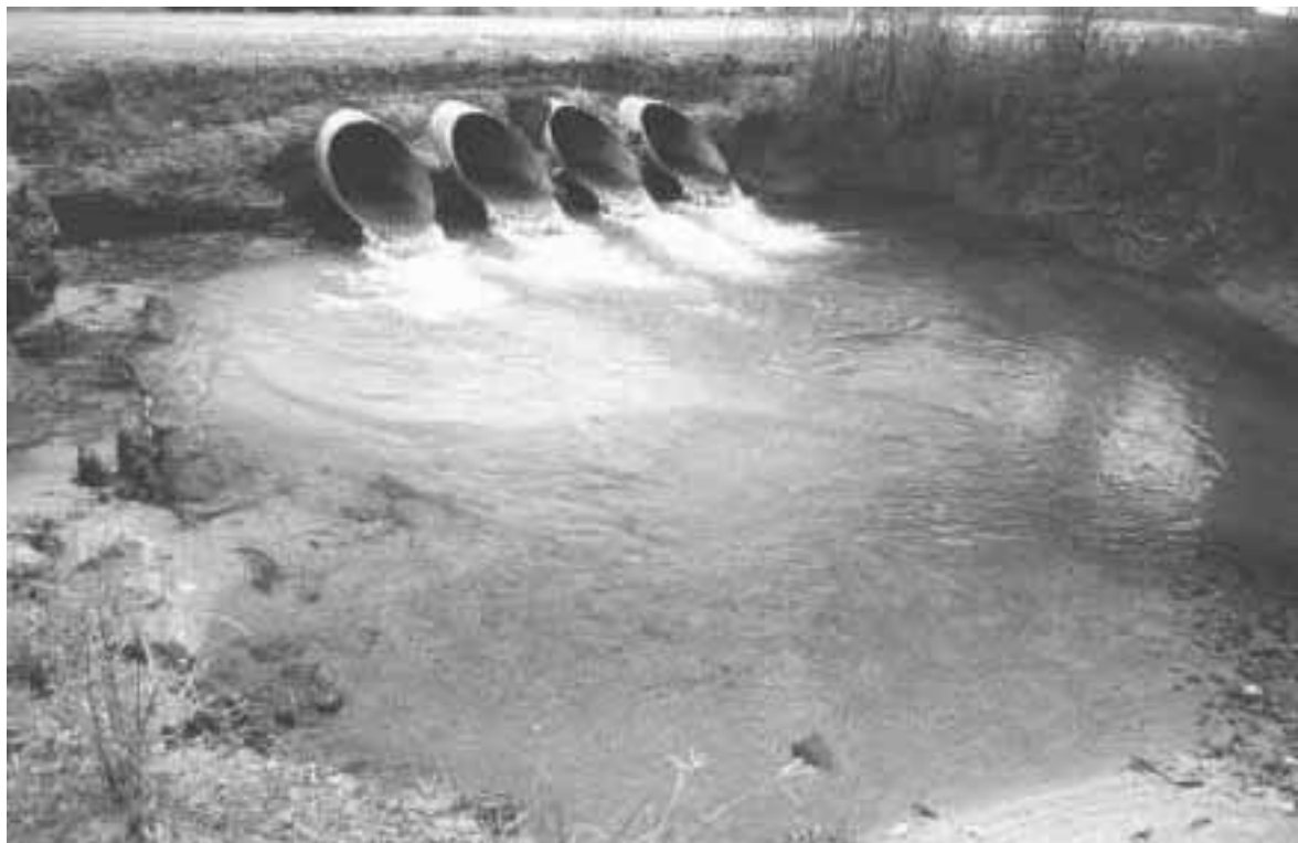
Figure 3. Installation of culverts of insufficient size has resulted in erosion in the vicinity of the outlet, creating a large scour pool. Tully, Queensland.
