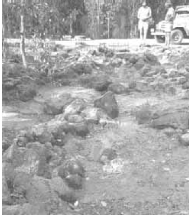
Figure 19. Rocks or boulders may be concreted on the downstream side of a causeway to reduce water velocity. Weipa, Queensland (Photo courtesy D. J. Russell).
