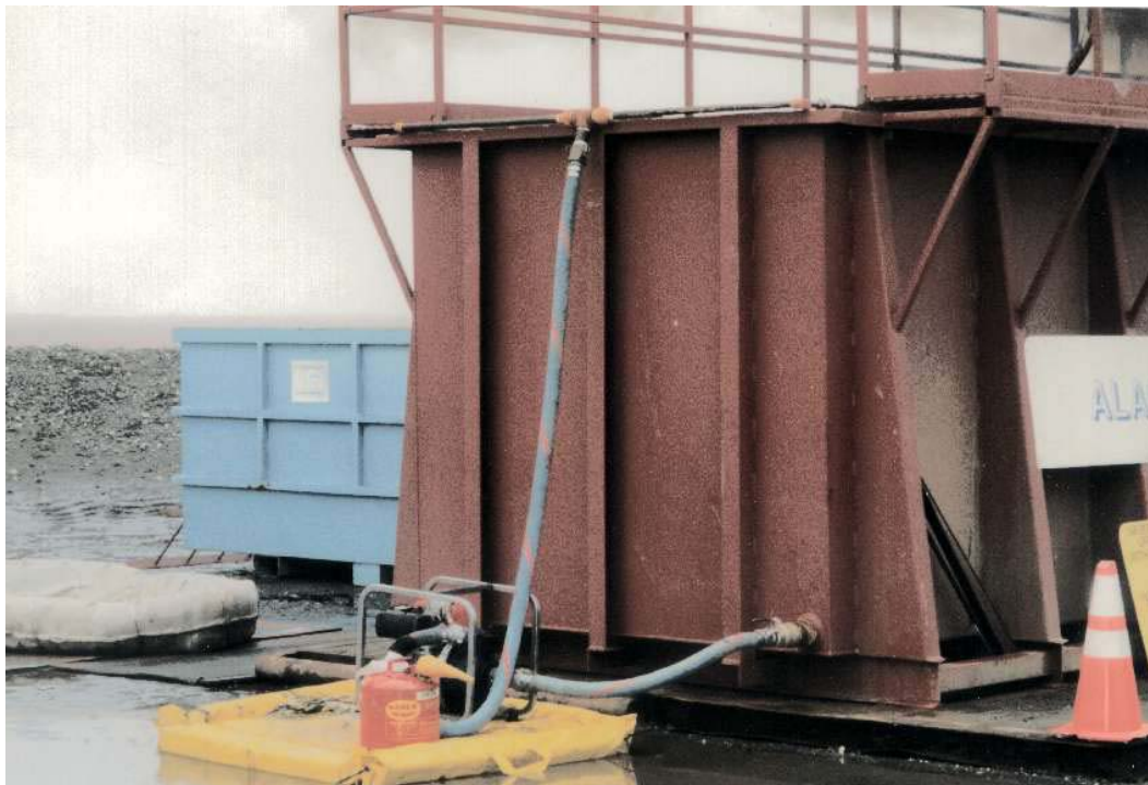
Figure 4-6: Pump system to feed water to deluge pipes along tank walls (see above picture).
