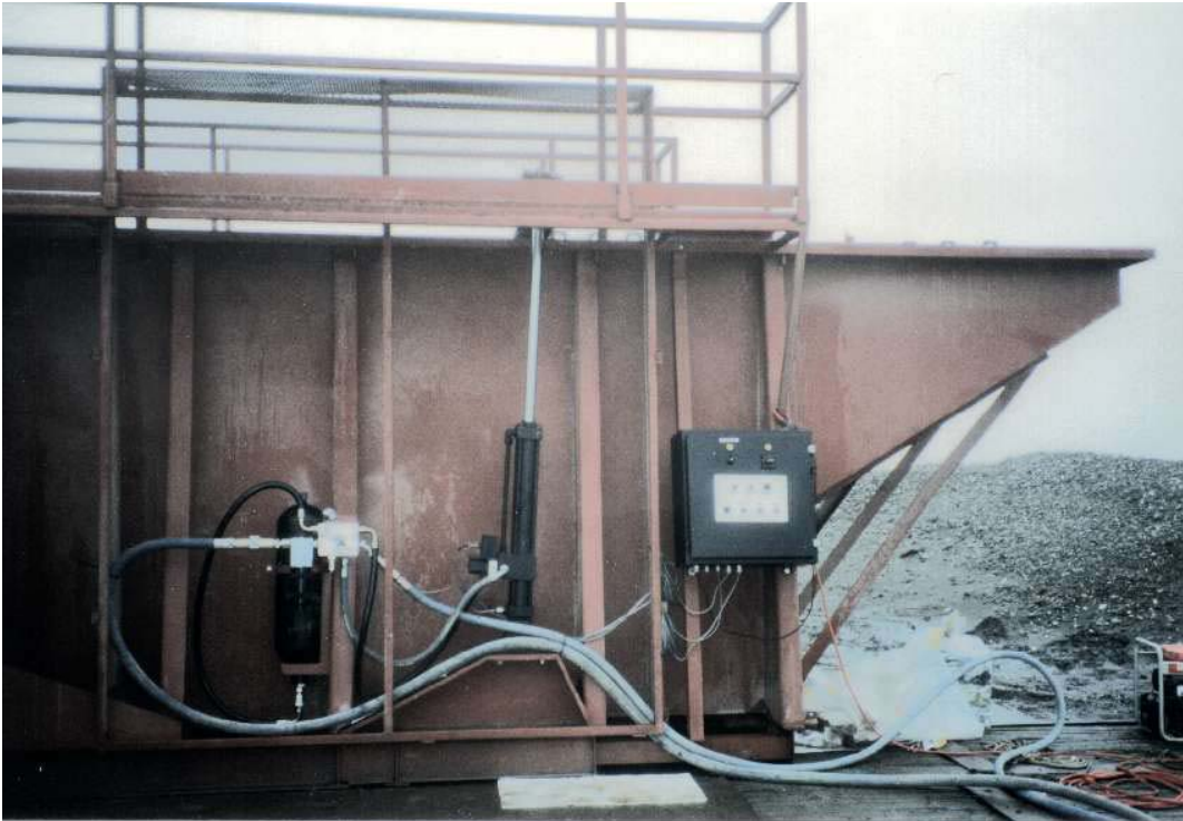
Figure 4-4: Electronic control panel and hydraulic drive system for wave board.
