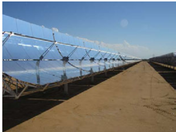
Fig. 1. New APS solar power plant using Solargenix parabolic trough concentrator and Schott receiver
