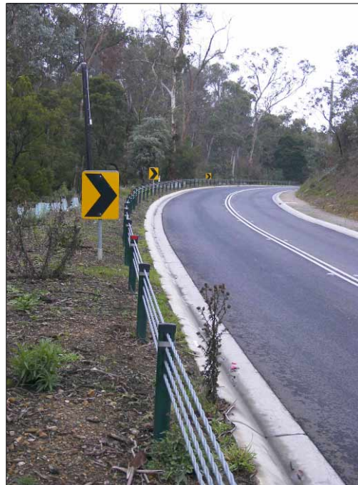
Figure 20 Four rope wire rope barrier
