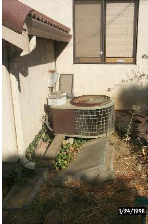
A good candidate for replacement: an old condensing unit showing poor condition of unit (heavily corroded sheet metal and fasteners and significant dirt/dust blocking flow into coil) and subsided slab (that we believe led to stresses on refrigerant lines with a subsequent leakage of refrigerant – this system had too little charge)
