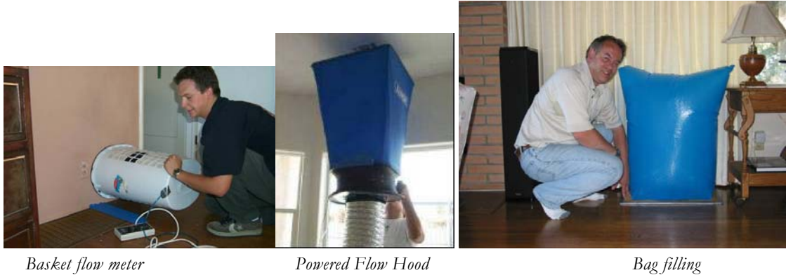
Various methods of measuring air flow at registers
