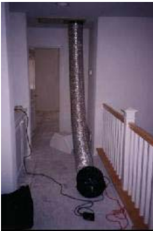
Duct pressurization uses a combined fan/flowmeter to pressurize a duct system to measure the flow through the leaks at fixed conditions
