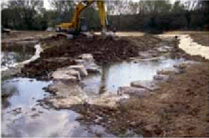
Beaver Creek project after channel was restored to original location and size, and streambanks were sloped back to provide a more stable vegetated area for higher stream flows.
