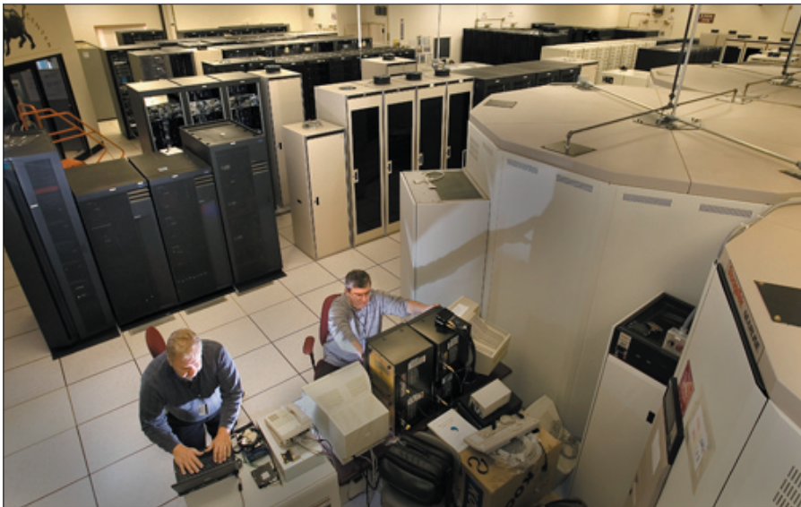
A bird's eye view showing part of the multi-million dollar RHIC/ATLAS Computing Facility, with Ognian Novakov (right) of the Physics Department and Jim Burkavage of Sun Microsystems monitoring the performance of the 7-petabyte robotic tape storage system.
