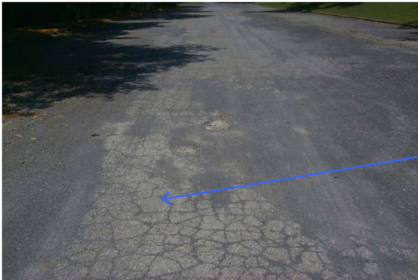
Upper Parking Area ● Cracking of the Pavement
