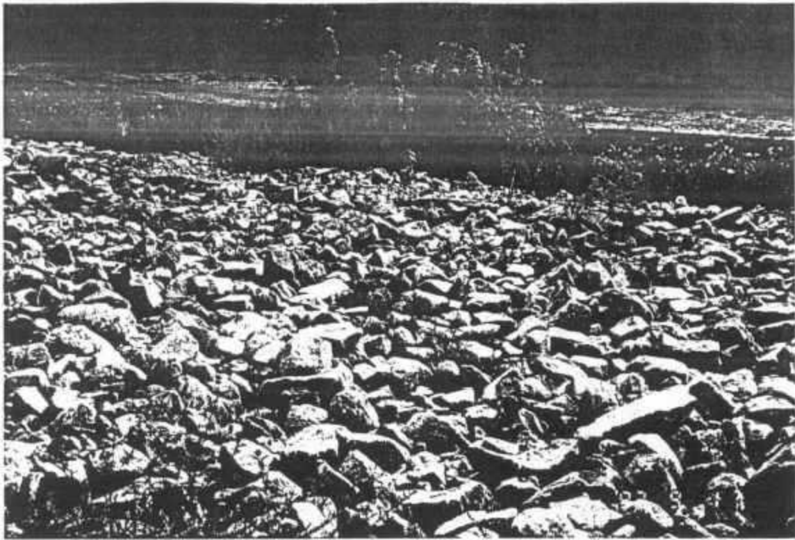
Photograph No. 5 Date: September 1, 1992 Location: Triana/Tennessee River, Triana, Alabama Description: View of Diversion Structure No.1 of the HSB showing rip-rap and sheet piling.
