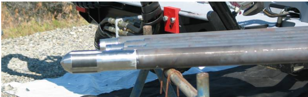
Figure 5.3. Cone-tipped Drive Shaft Used in Conjunction with a Hydraulic Hammer for Creating Driving Boreholes
