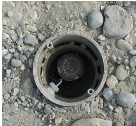
Figure 5.4. Capacitance Probe Cap and Protective Casing at Instrument Nest B Before Filling With Tank Farm Surface Material
