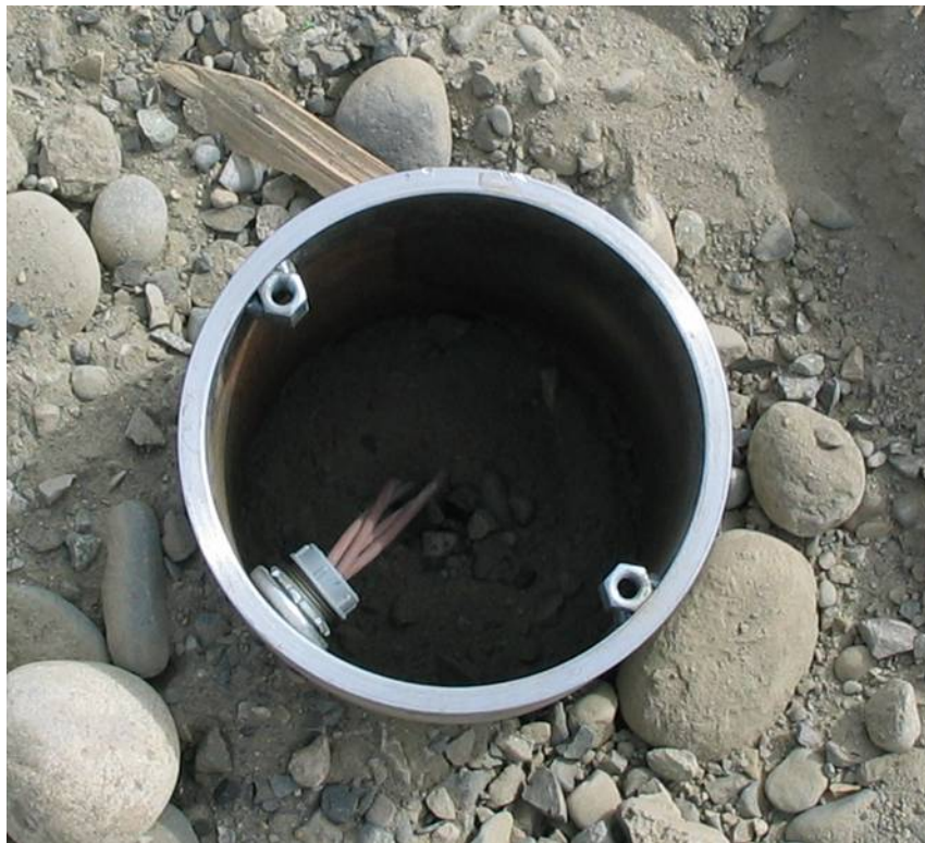
Figure 5.6. Protective Casing Over the HDU Location at Instrument Nest B
