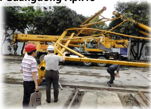
Gantry crane collapse in Guangdong Apr.13
