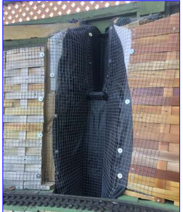
Preparation for the top half of the waterfall with the pool liner held in place by the wire netting
