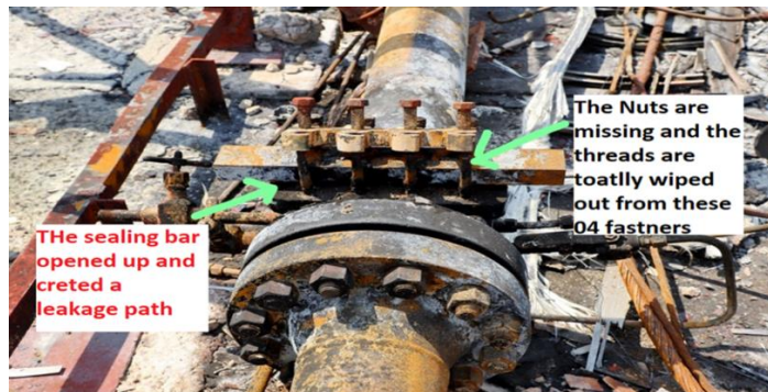
Source of leak
