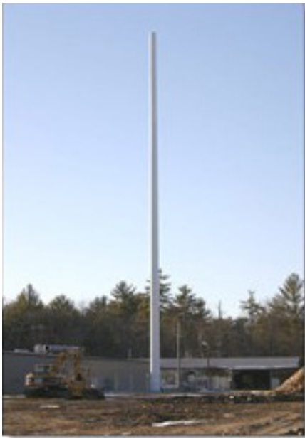
Example of Monopole Tower
