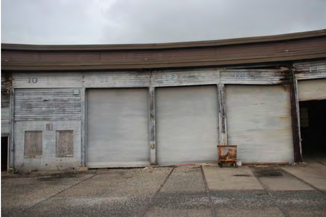
Bays #10 to #14. Note bays #11 to #14 still have their track in place and overhead doors that work.
