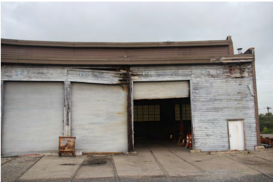
Bays #12 to #15. While all have their track in place, only bays #12 to #14 have doors. All of these bays still have their drop bits in place.
