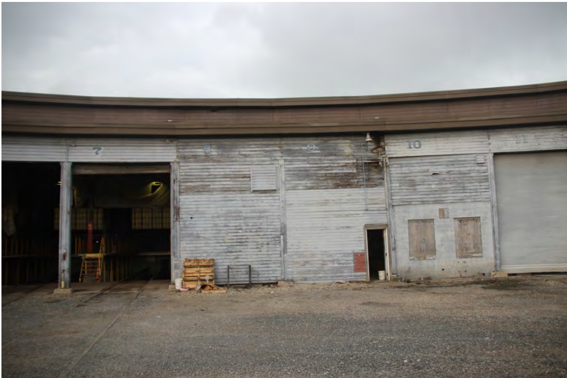
A view of bays #7 to #11. Note bays #8 to #10 are sealed and their access track removed.
