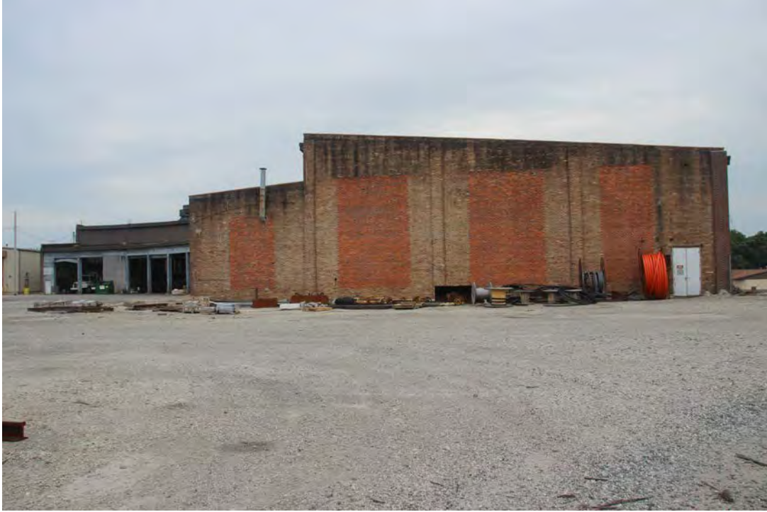
A view of the rear of the right side wall of the roundhouse
