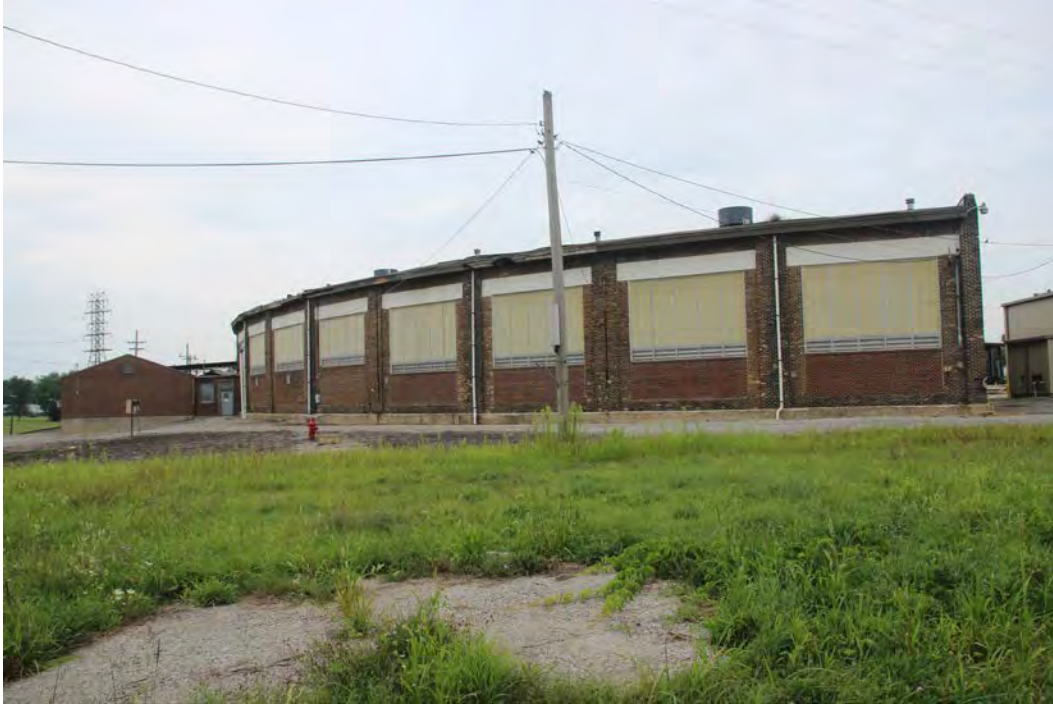
A view of the rear of the roundhouse looking at bays #1 to #7
